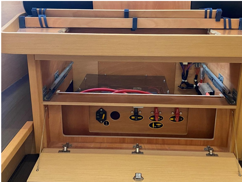
Figure 4: 800Ahr installed Lagoon 450F/S
