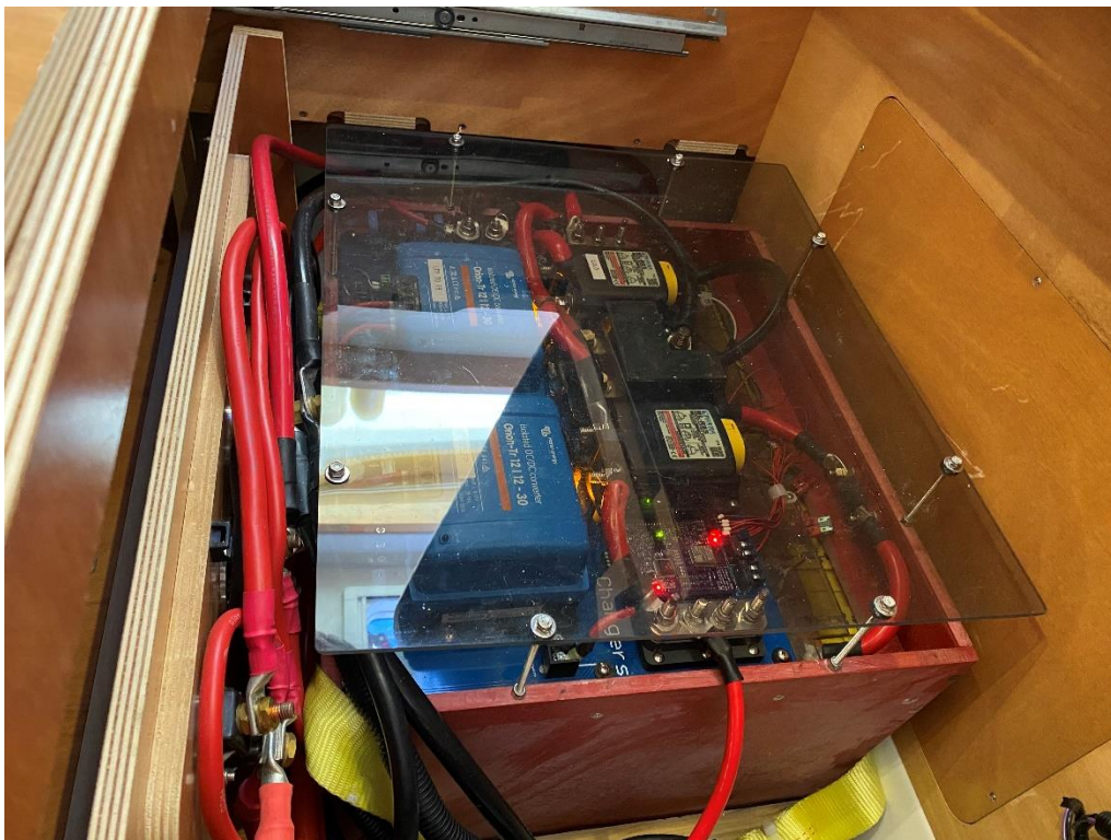
Figure 3: 800AHr installed Lagoon 450F/S
