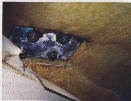
The woefully inadequate backing plate was pulled right up through the GRP
