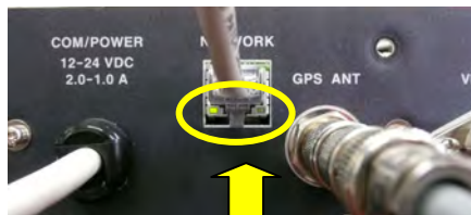
LAN connection check
